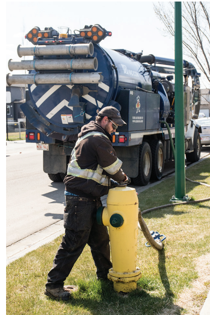
Left: Employee Justin Sinnett accesses the municipal water supply to fill a Vac-Con combination truck being used on a cleaning job.
